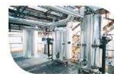
Wet Oxidation Plant Porto Marghera - Italy
